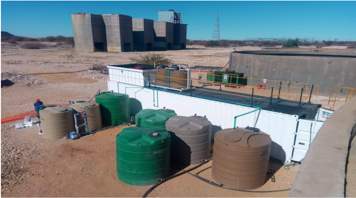
Figure 2: Water treatment plant container and processing tanks at the Prieska Project site.
