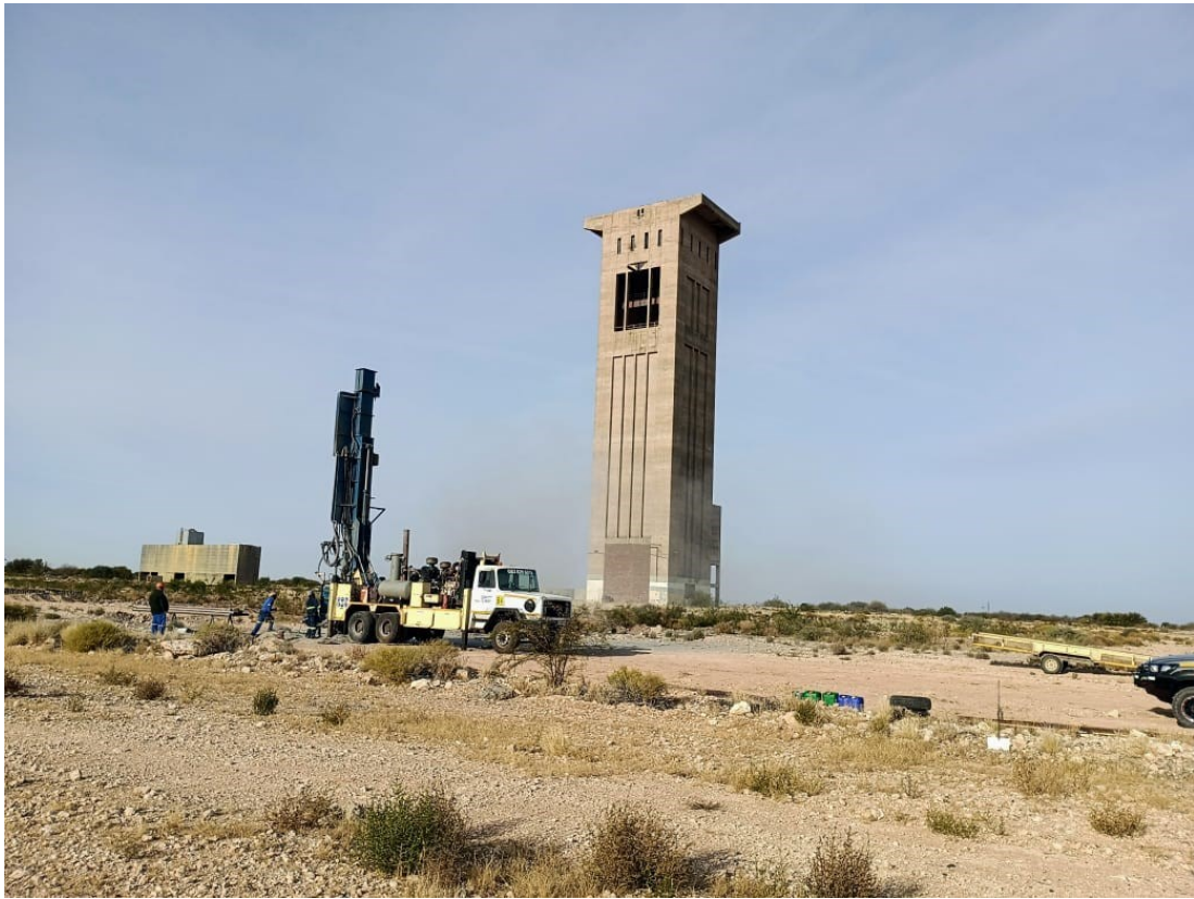
Figure 1: Drilling in progress for installation of rising main pump column from the 178 level.
