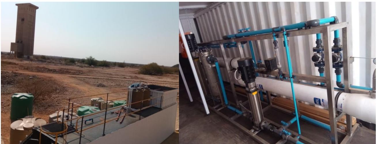
Figure 2: (LHS) Water treatment pilot plant mobilisation. (RHS) Commissioning the chemical treatment, ultrafiltration and reverse osmosis components of the pilot water treatment plant, setup to operate at 5m 3 /hr of feed water.
