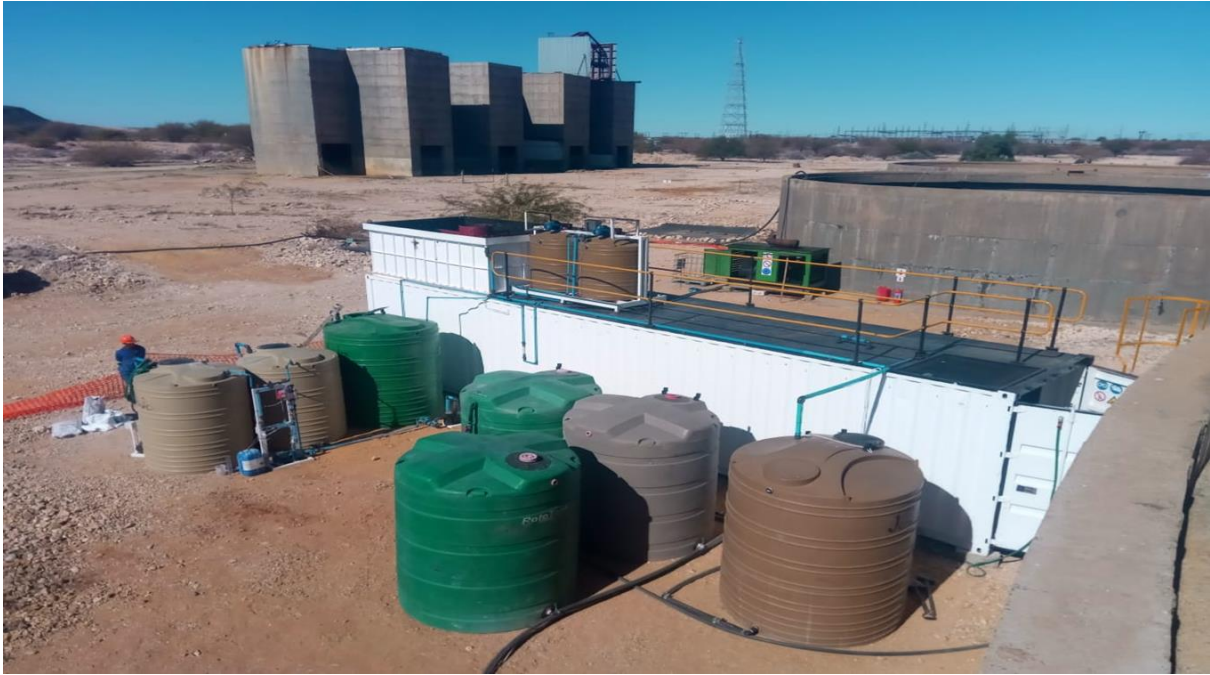
Figure 3: Pilot scale containerised water treatment plant and processing tanks at the Prieska Project site.
